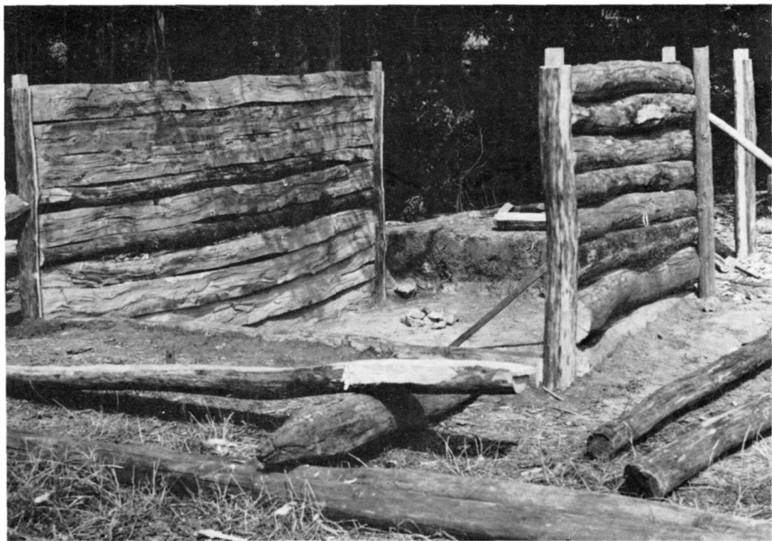
Fig. 15. House No. 69. 1 — work on a half - round timber tenon; 2 — building of E and W walls of half-round timbers inserted into post grooves.
